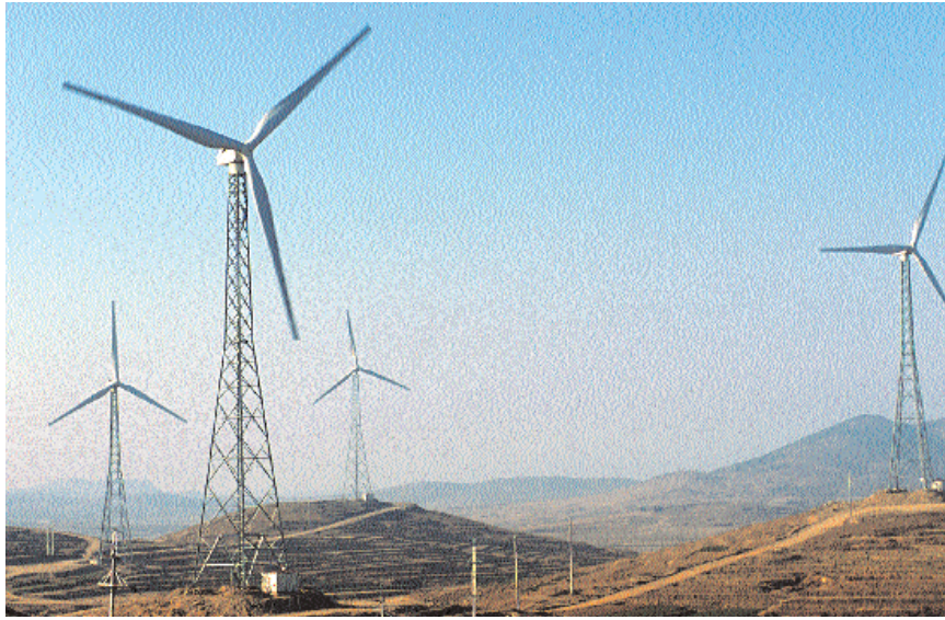
1.3 MW turbines installed at Qingdao NORDEX
