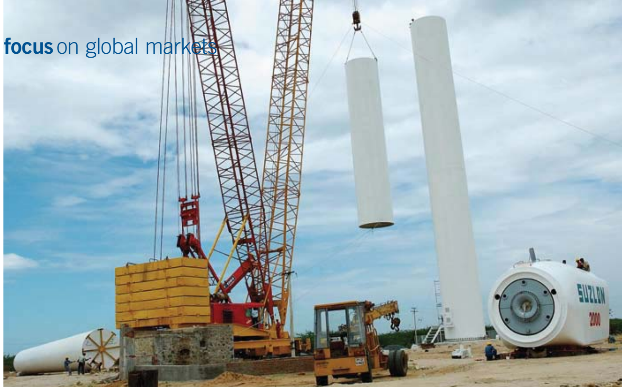
Indian market leader: Installing a Suzlon 2 MW turbine and (below) manufacturing Suzlon turbines at Pondicherry
