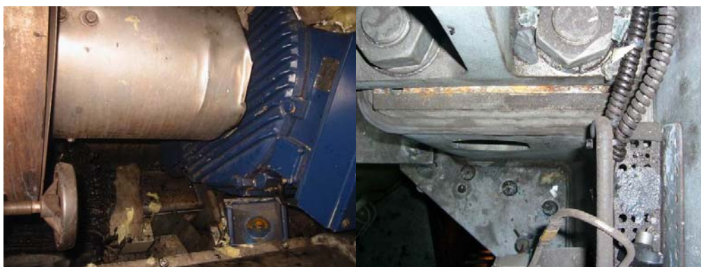
V42 generator base feet broken and main bearing seats displaced
