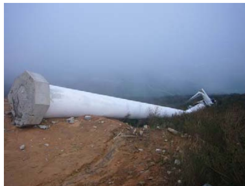
Whole wind generator fell after foundation failure
